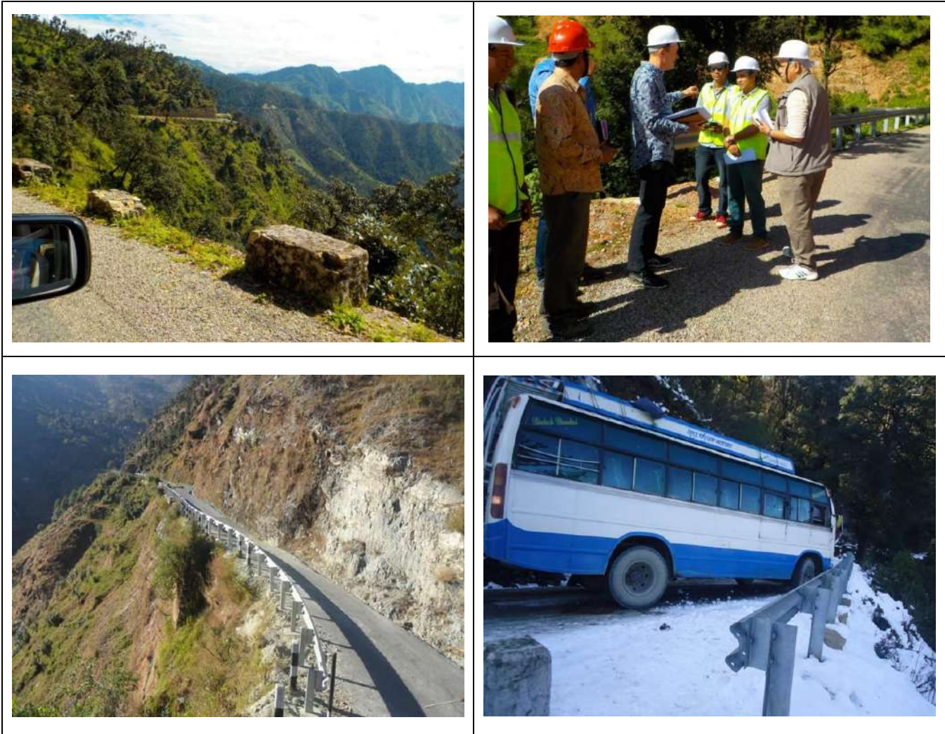
Figure 4.4: Roadside Barriers in Nepal. The GRSF funded construction of roadside barriers on cliff-side roads in Nepal, showing in order the road without barriers, during construction, at completion, as well as an example of a bus which was prevented from going over the cliff by the barrier
